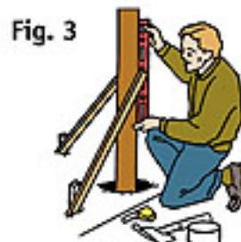
Use a level to make sure each post is in an exact, upright position.
